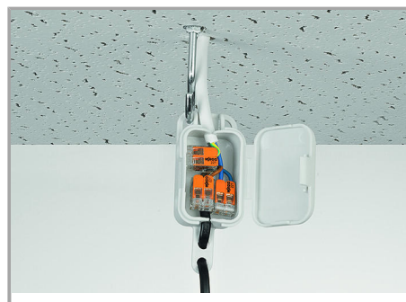
Pendant light connection in suspended ceilings
