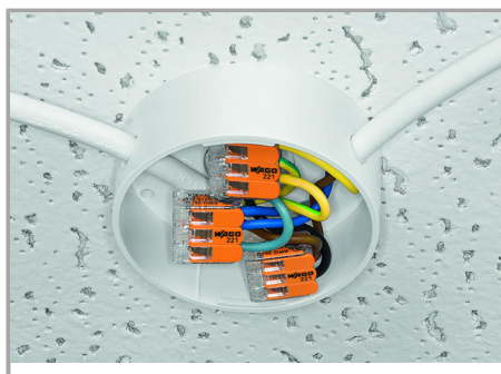
Lighting distribution in ceiling canopy
