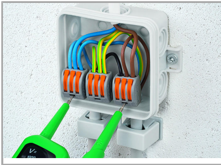
Testing via Profi-LED+ voltage tester (206-806).
